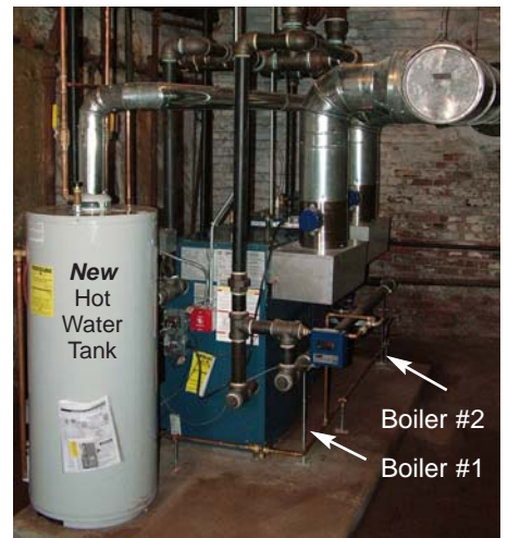
Boiler #1 will heat the Church Boiler #2 will heat the Office, Noah's Ark Rm., Gym, Parish Hall, and Kitchen
